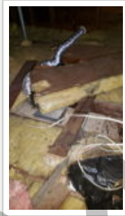
The bath fan is poorly vented as it dips down in between bays in the attic and is not insulated allowing condensation in the rigid vent. This vent should be revented without any dips and properly insulated.
